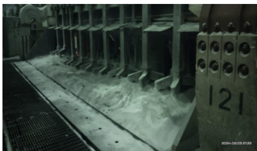
Figure 14. Pilot cells anode cover condition with redressing practice.
