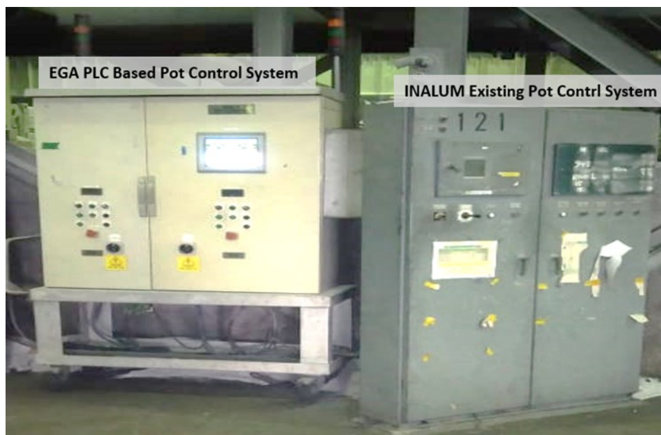
Figure 4. EGA Pot Control System (left) replaced INALUM Pot Control System in pilot cells.
