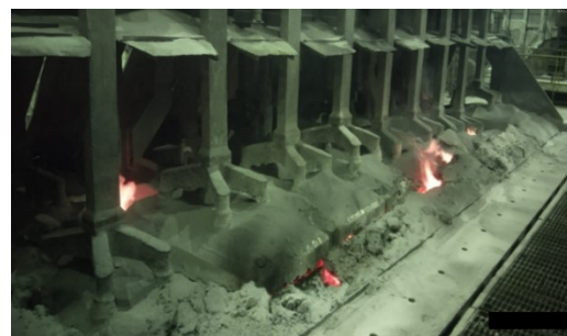
Figure 15. Existing cells anode cover condition without redressing practice.
