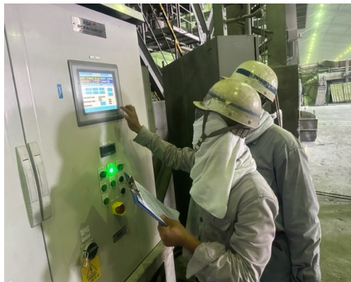
Figure 9. Data entry of cathode surface temperature into HMI.
